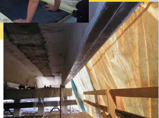
Eight weeks after the workshop, Perm engineers had the CFRP laminate in place on the Tiskovka Bridge.
