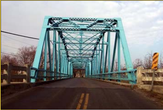
The old steel bridge over the Licking River in Pendleton County was built in 1928.
