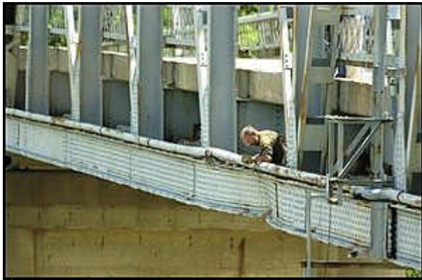
A state inspector surveys the damage to the bridge.
